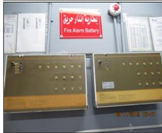
Photo of fire safety equipment Fire alarm panel.JPG
