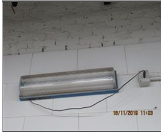
Photo of the inside of the main production hall Emergency light.JPG
