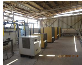
Photo of the inside of the main production hall Compressors room.JPG
