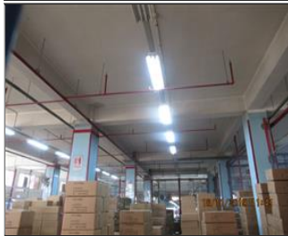
Photo of fire safety equipment Sprinkler system - warehouse.JPG
