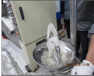
Photo first aid facilities Eye wash station - washing section.JPG
