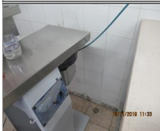
Photo of non-conformity Fumes from stain removing table not exhausted to the outside.JPG
