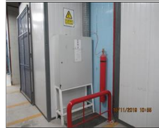
Photo of fire safety equipment Fire extinguisher.JPG
