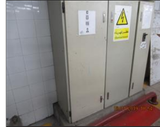
Photo of the inside of the main production hall Electrical panel.JPG
