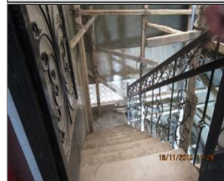
Photo of non-conformity Emergency exit staircase under construction.JPG
